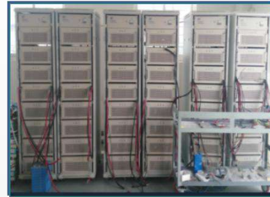
Battery charge and discharge test
